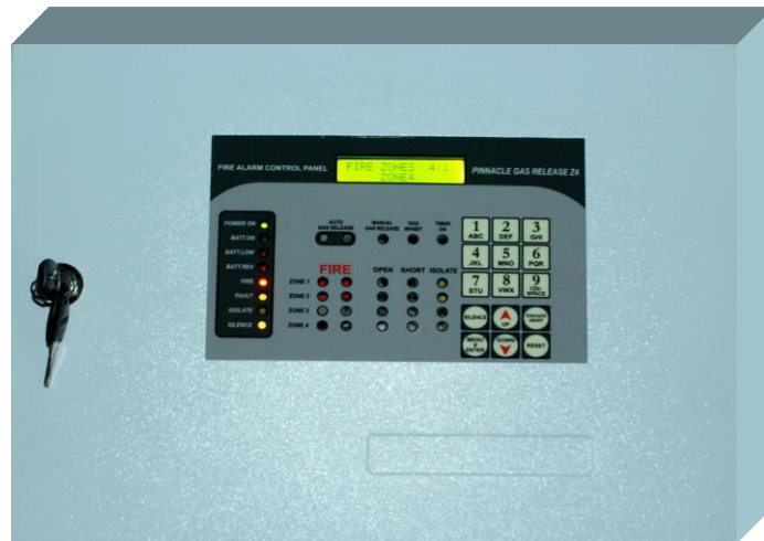
2Z-4 ZONE GAS RELEASE PANEL
